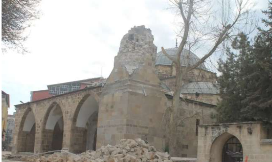
Figure 1. Collapsed masonry minaret of Ulu Mosque in Elbistan, Kahramanmaraş (İlkha 2023)
