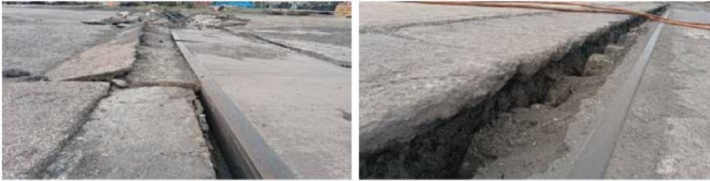
Figure 5. Fracture and Collapse Identified at Iskenderun Port After the 2023 Kahramanmaraş Earthquake
