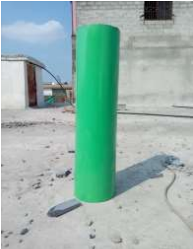
figure 2.3 PVC pipe Green spray paint coating
